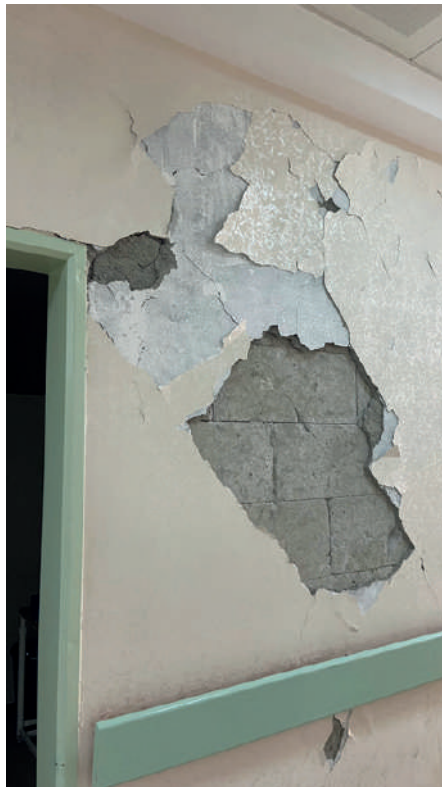
Picture 2. Hospital walls after earthquake
